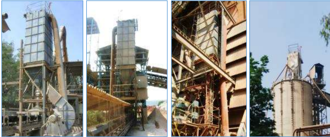
Bag filters at various material transfer points & silo top
