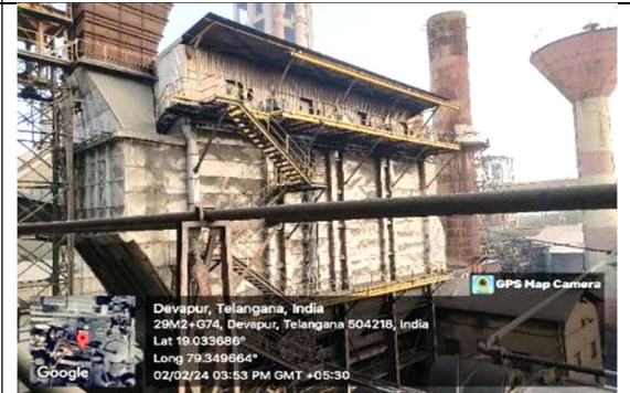
ESP for with stack Clinker Cooler – Line2
