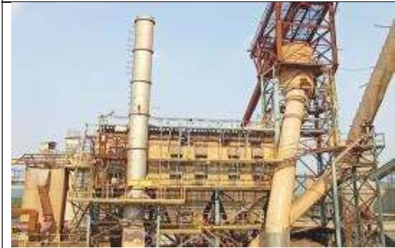
Coal Mill -1 VRM Baghouse
