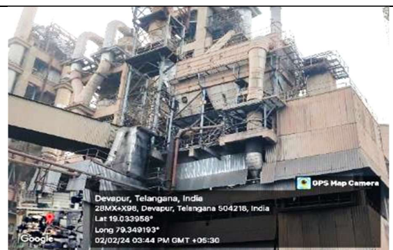
Bag House for Coal Mill VRM – Line1
