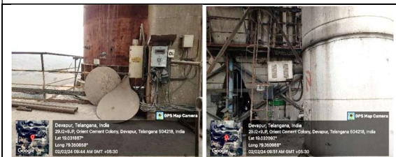
CEMS at Kiln-3 Stack & CEMS at Coal Mill-1 Stack
