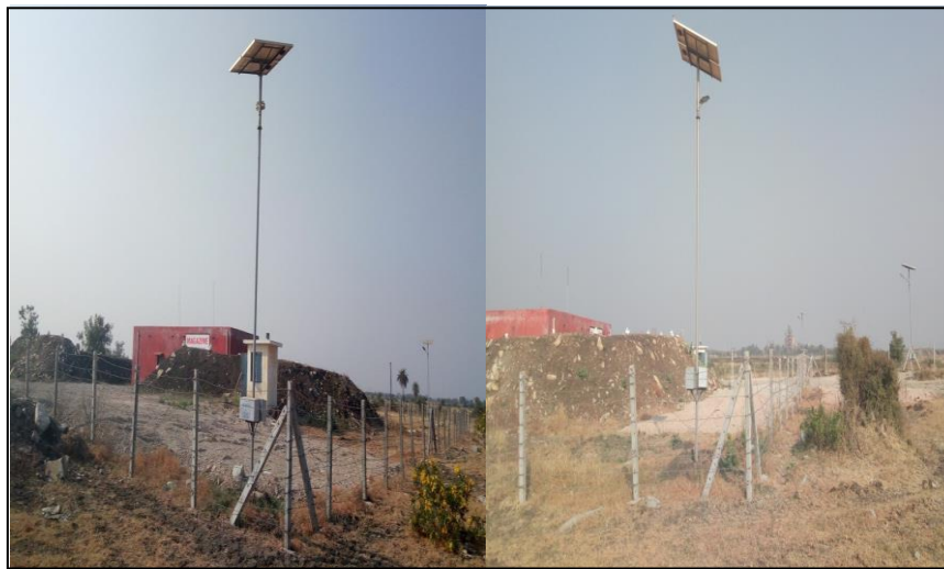
Arrangement of Solar light Panels in required areas
