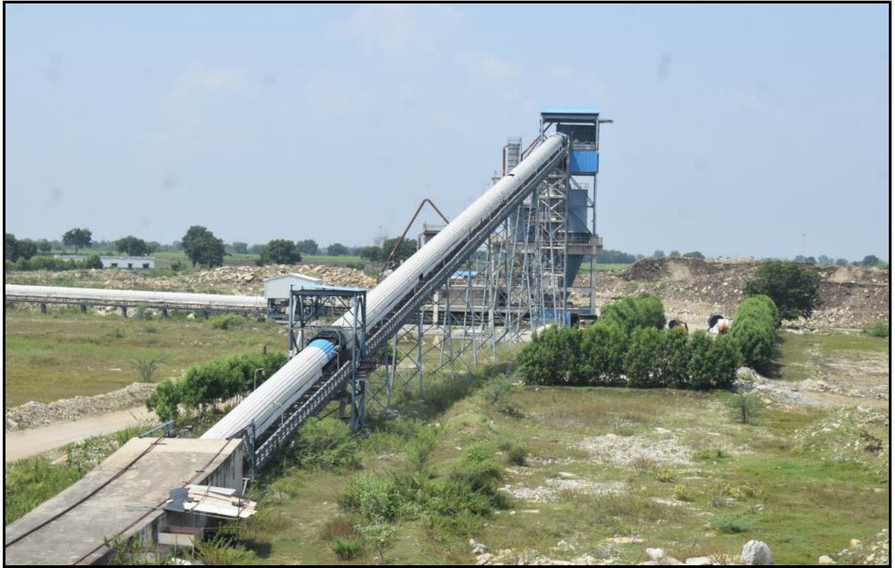
Closed Belt Conveyor
