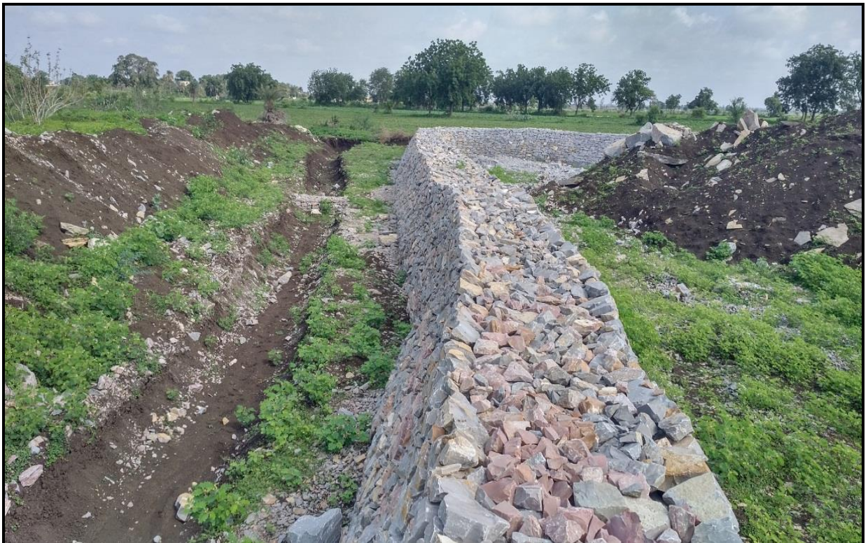
Garland Drain along the Dump Toe Wall with Random Rubble Barriers
