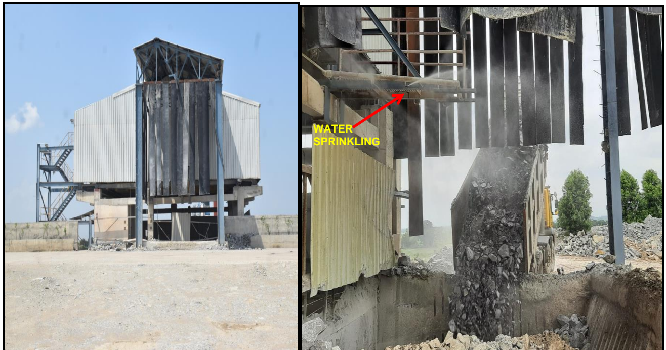
Rubber curtains & Water sprinkler system provided at Limestone dump hopper to Control dust at Lime stone Crusher
