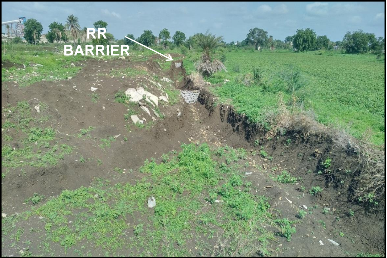
Garland drain with RR barrier
